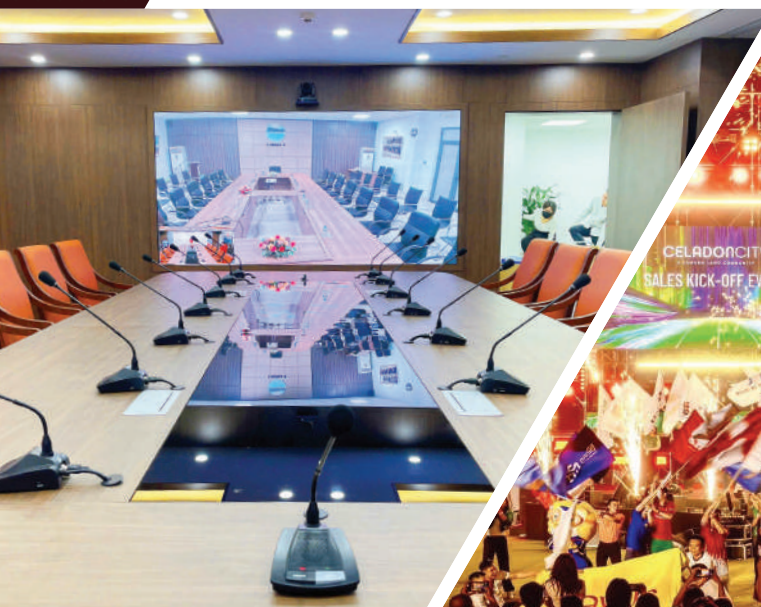
PA SYSTEM, COFERENCE SYSTEM
